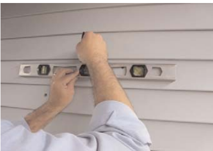
DRILL (4) 1/2" CORNER HOLES THROUGH WALL FROM INTERIOR AND CONNECT HOLES ON EXTERIOR WITH A LEVEL. ALIGN TEMPLATE WITH HOLES AND TRACE REMAINING LINES.
