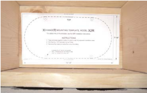
CENTER AND LEVEL TEMPLATE BETWEEN JOISTS / TRUSSES OR PLACE ON WALL X2R XCHANGER WILL EXIT.
